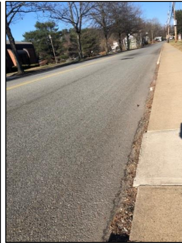
Curbing is crumbling, missing, damaged in sections after Pocono Road intersection
