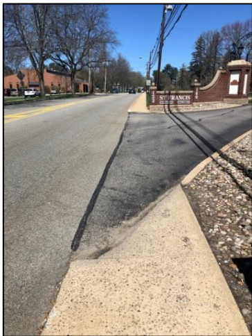
Sidewalk does not continue across driveway at St. Francis
