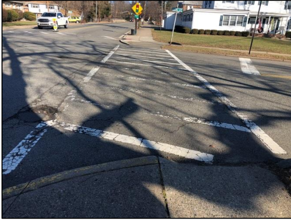
Faded crosswalk at 2 nd Avenue and no truncated dome/ADA compliance
