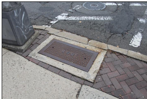
DOT utility plate where a truncated dome should be
