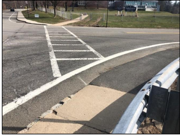
Lack of ADA infrastructure at the middle school
