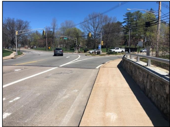
Pocono Road intersection crossing is hard to see
