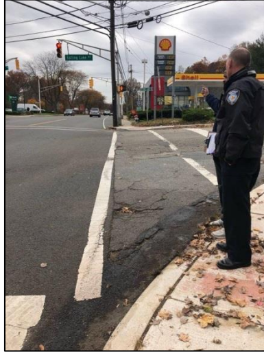
Estling Road crossing lacks a buffer for pedestrian at corner
