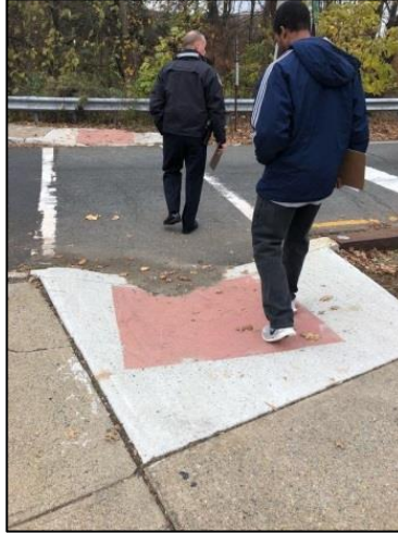
Curb ramp is painted not a truncated dome
