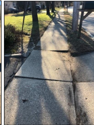
Cracked and uplifted sidewalk
