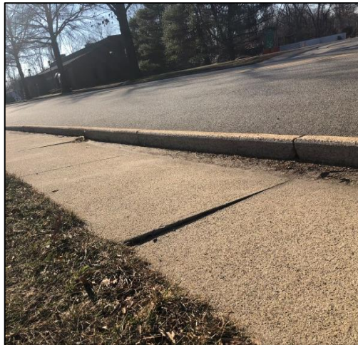
Sidewalk is sunken down and curb is raised along Diamond Spring Road
