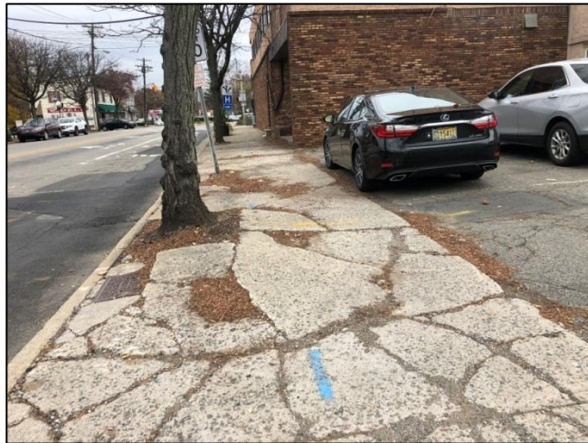
Cracked sidewalk on the north side of the road and a lack of buffer between the parking lot and sidewalks
