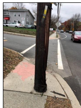
Chipped pole at Cooks Road
