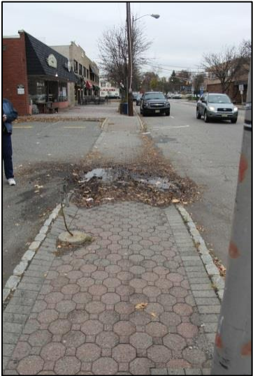
Cracked pavers and water retention along East Main Street
