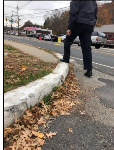
Lack of ADA compliance with no curb ramp or truncated dome
