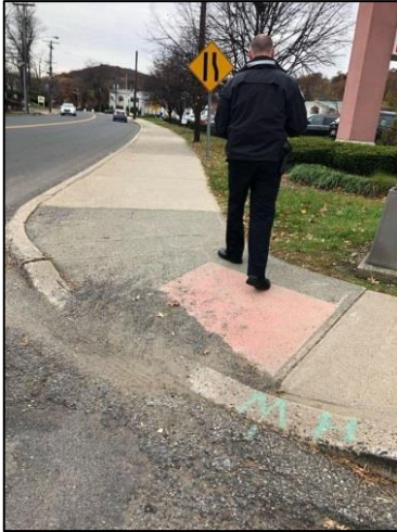
Curb ramp is painted no a truncated dome, is covered by debris, and a steep slope
