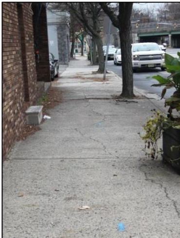
North side of the road is wide but is in needs of maintenance
